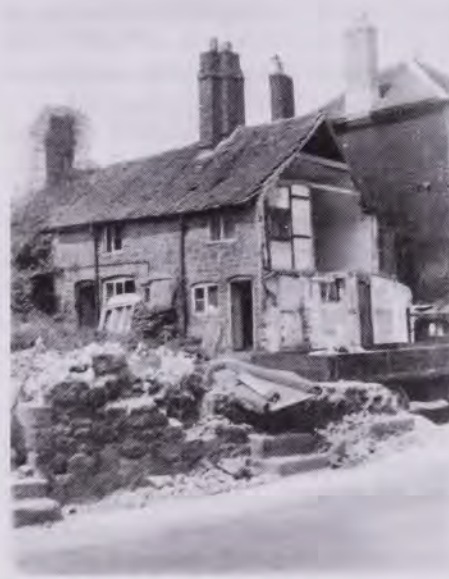
Demolishing old cottages in Pound Street 1962. The buildings at the front have been demolished: this shows the cottage to the rear.
