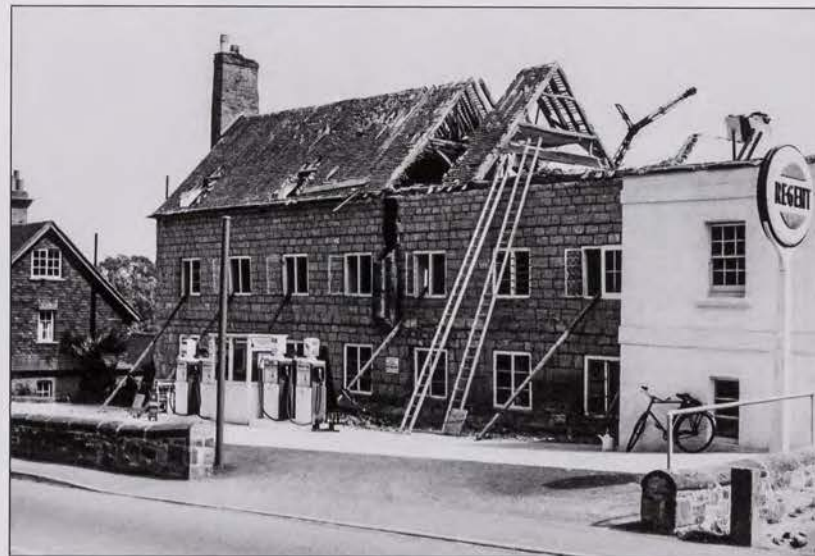
Demolition of the old workhouse premises in 1960, considered the most "beautiful" workhouse in Sussex after that at Battle.
