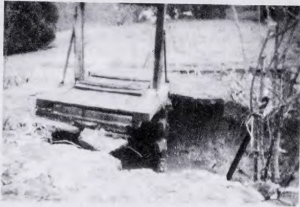
Collapsed well at 'Potters' Bedham.
