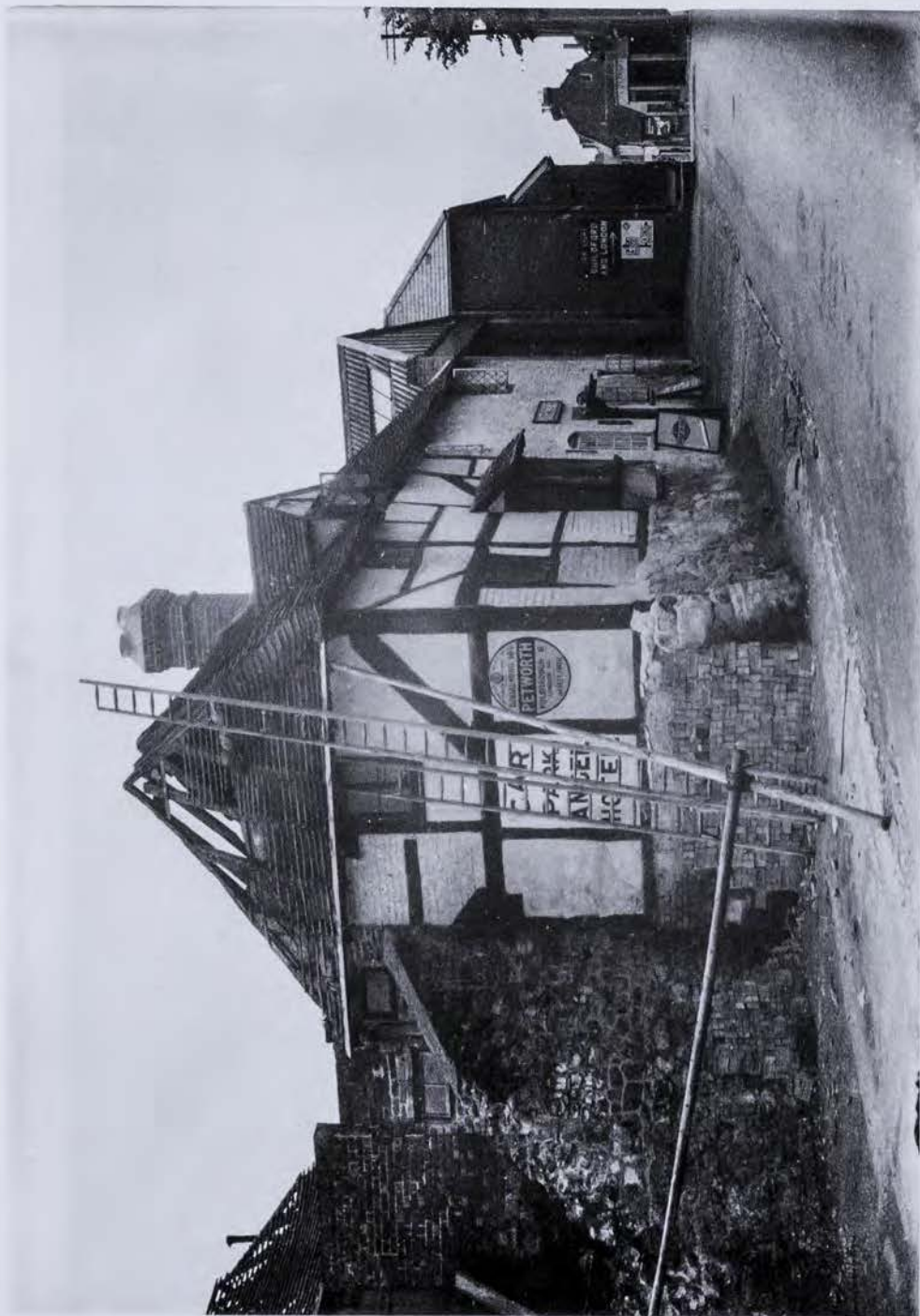
Demolition of old cottage in Angel Street July 1939. (Photograph by George Garland.)
